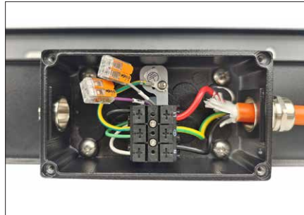
Terminal block showing simple DC wiring for dimming via Wago connectors.
