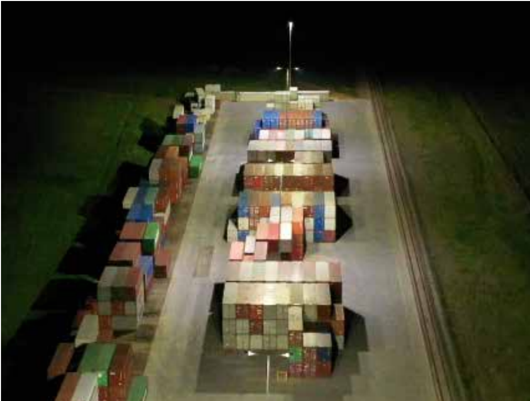
Left: Uniform light spread along the hard-stand area. Minimal light spill into surrounding areas, due to the anti-spill lens design, unique to Tigerlight's MEGA floodlights.
